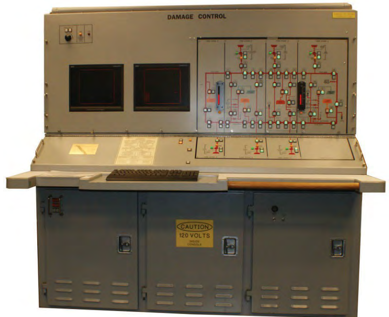
Figure 6-31 — Damage control console.
