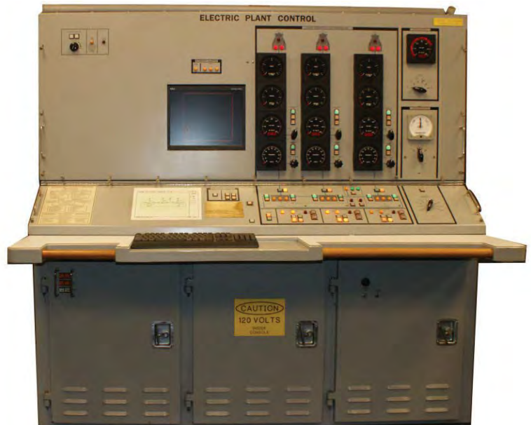
Figure 6-28 — Electrical plant control console.
