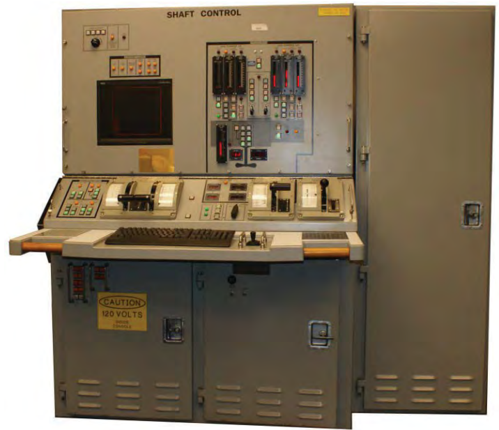
Figure 6-30 — Shaft control unit.
